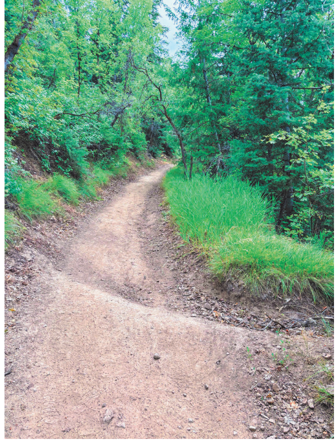
Water bars across the Switchbacks are necessary to push water off the trail.
